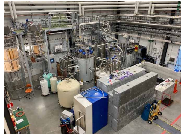
Figure 2: FREIA hall – liquefier and vertical cryostat.
