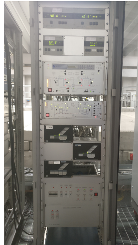
Figure 1: One of the TELEMA racks mounted in ALPI.
