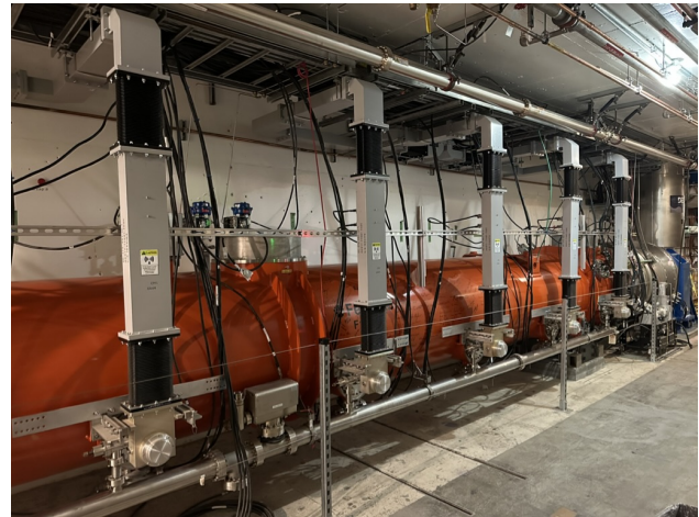
Figure 1: Photo of LCLS-II L0B cryomodule string.
