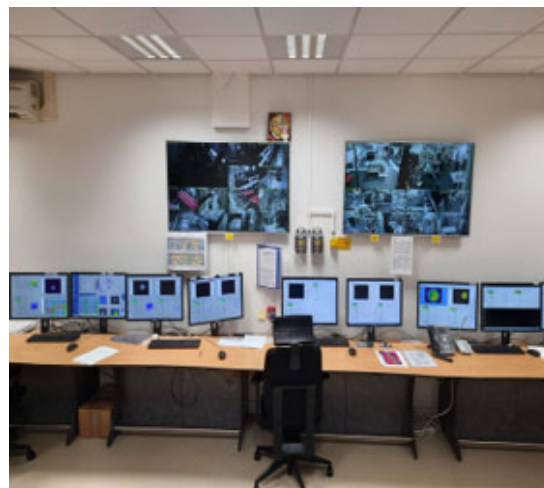
Figure 1: Supervision control room.
