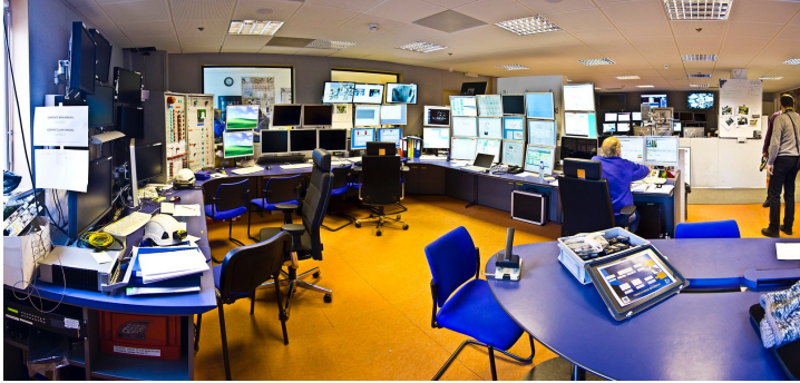
Figure 1: CMS control room
