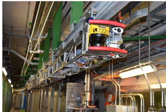
Train Inspection Monorail (CERN made)
