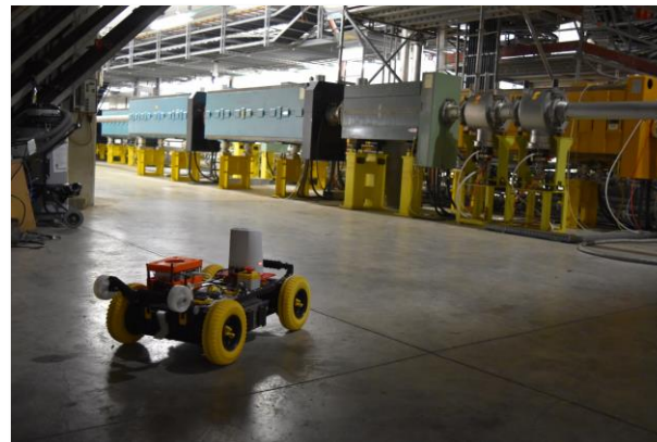
EXTRM robot (CERN controls)
