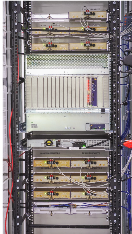
BPM/FOFB Rack Rear view
