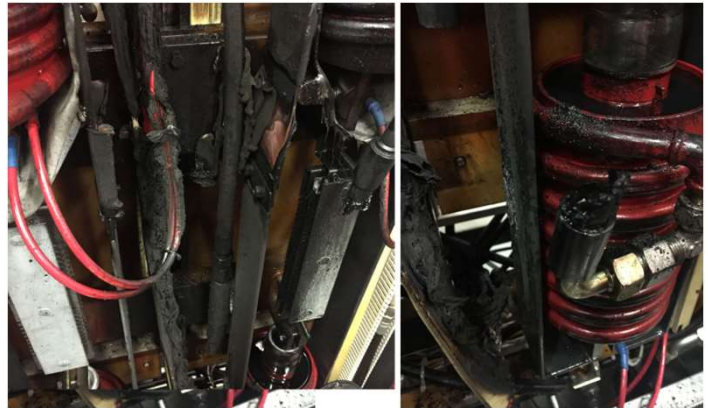
Fig. 1 - Aftermath of Fire in AD Horn Equipment Rack
