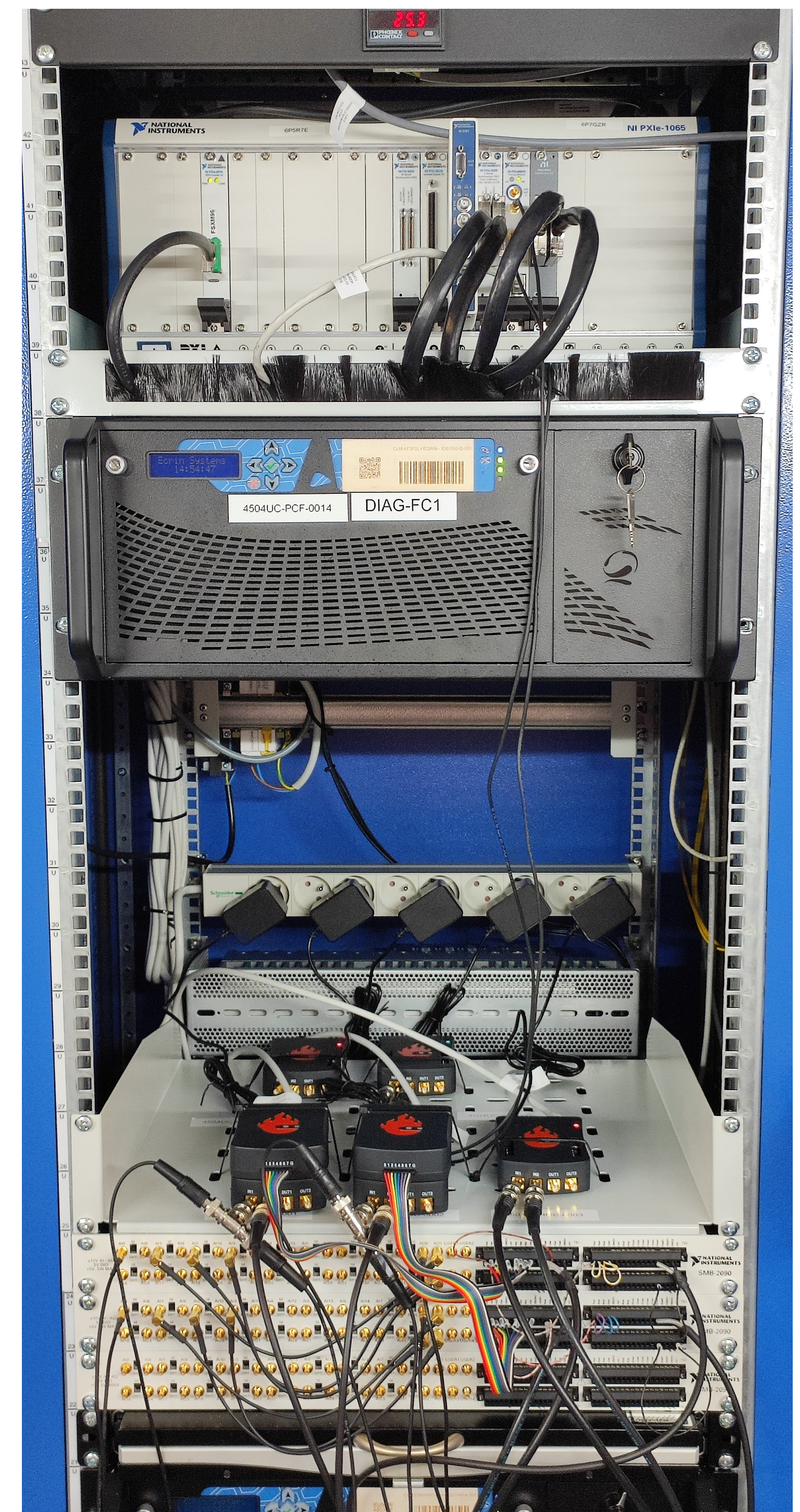
Test Stand: Fast Controllers.
