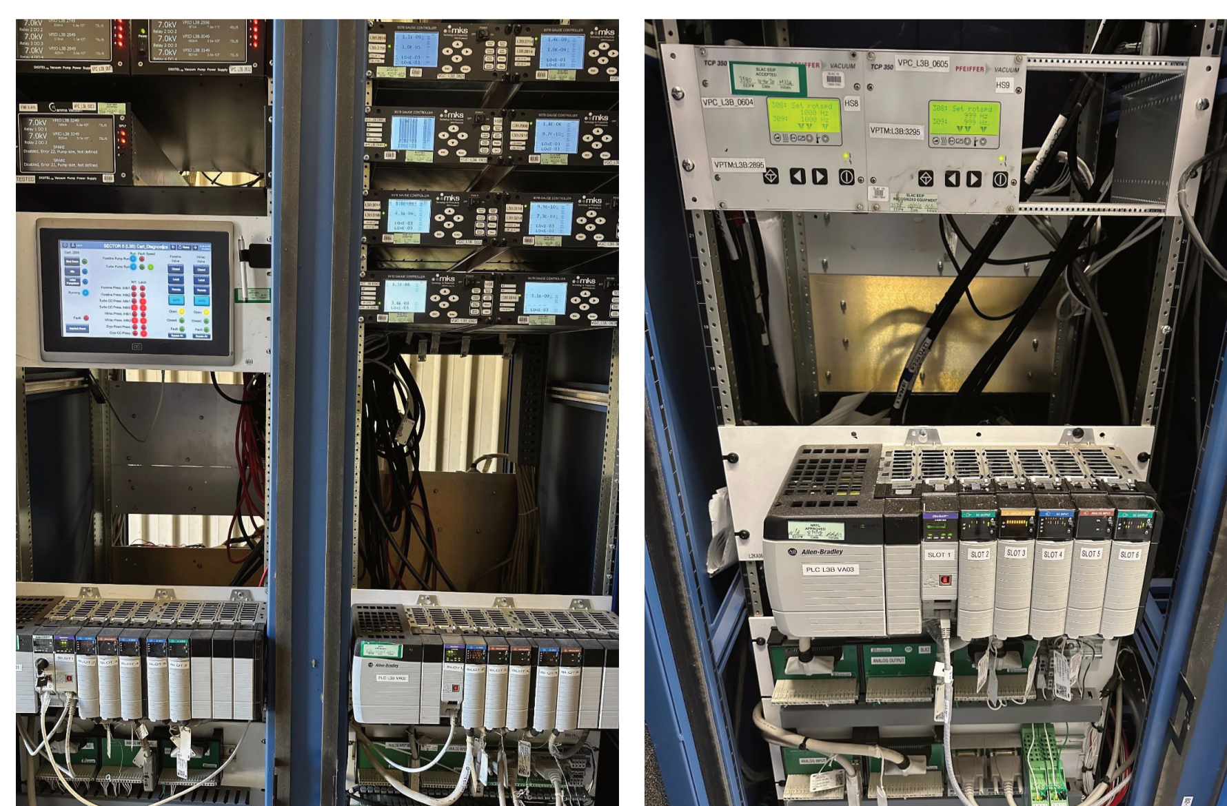
Shared ControlLogix PLC and gauge/pump controllers.
