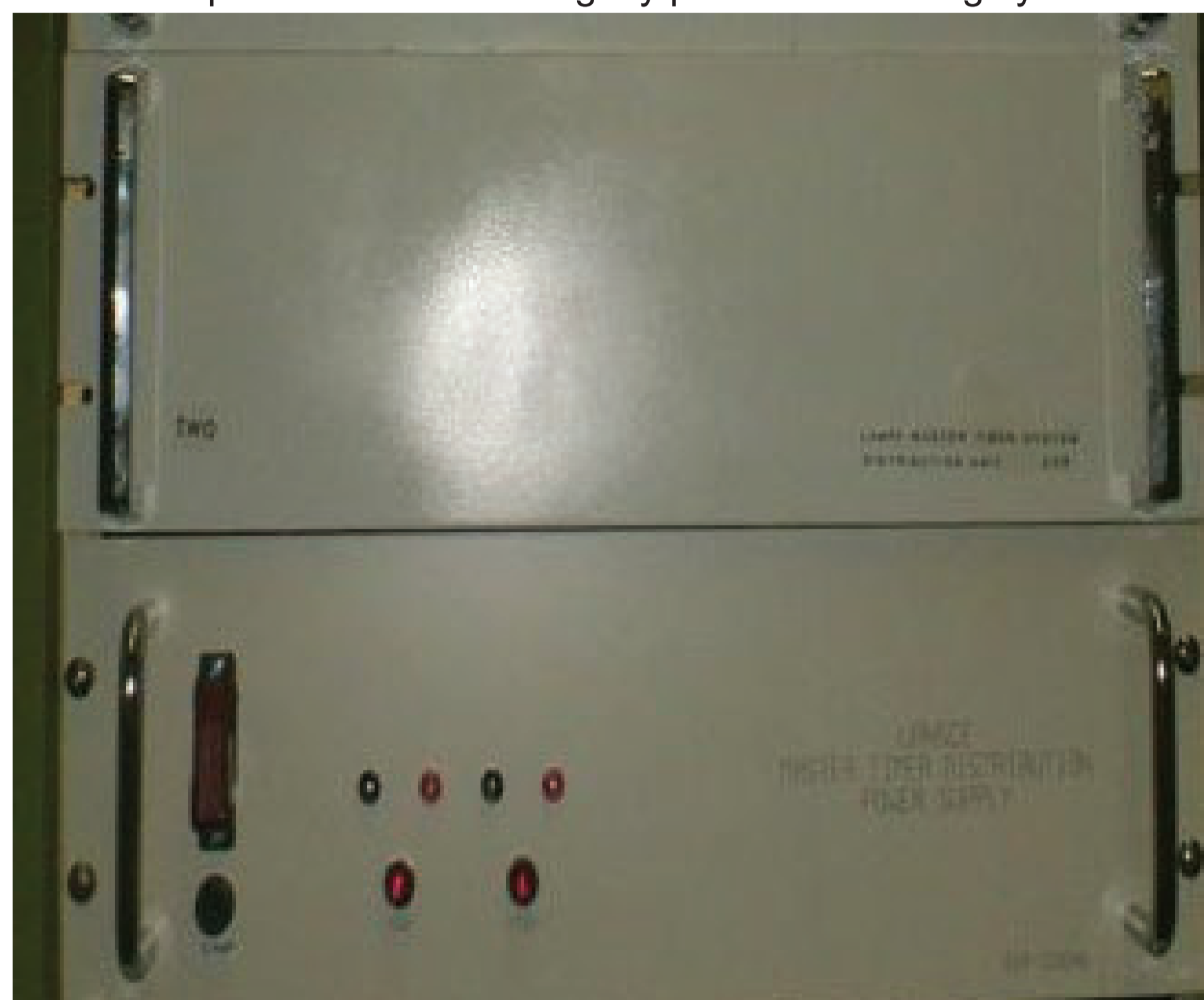
Legacy Timing Distribution Unit
