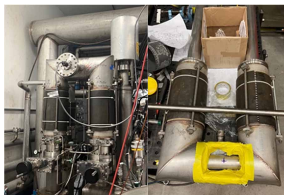
Figure 5: Sensor installed in the return U-Tube.
