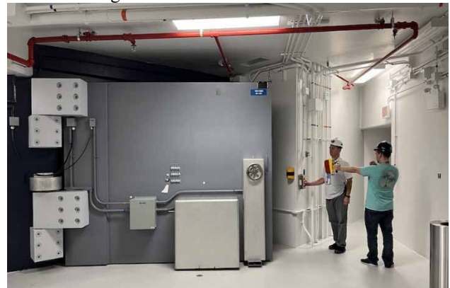
Figure 13: Massive concrete-filled Target Bay doors are opened after a high-yield experiment, under stringent radiation survey protocols.
