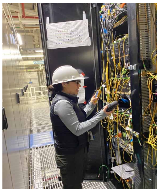
Figure 17: Maintenance of NIF diagnostics and cables in a switchyard rack.
