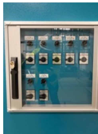
Figure 11: Test switches placed on front door of the TSS cabinets in Target Utility area.
