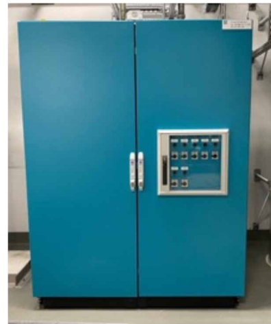
Figure 10: TSS cabinet in Target utility.
