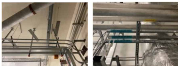
Figure 9: TSS metal cable conduits.
