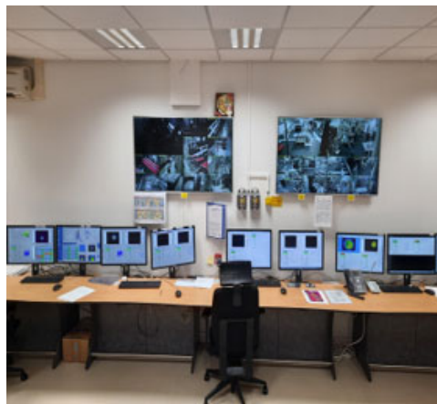
Figure 1: Supervision control room.
