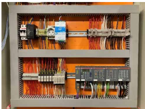
Figure 3: A photograph of an upgraded PLC.
