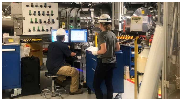
Figure 13: Controls team performing the Target Positioner SIS Periodic Test Procedure, which is a Configured Item and performed every 6 months for worker safety. Credit: Tom Kohut/LLNL.
