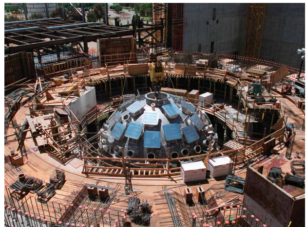
Figure 2: The 1999 installation of the NIF target chamber inside the half-constructed Target Bay. Credit: LLNL.
