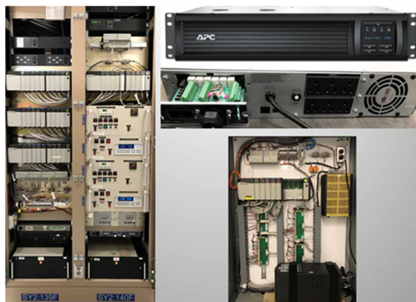
Figure 7: New UPS units and I/O cards in the Target Chamber Vacuum and SIS PLC racks/enclosures. Credit: LLNL.
