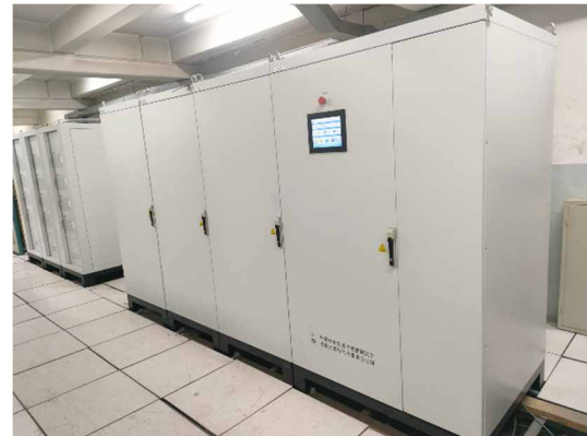
Figure 4: SFC power supply room.
