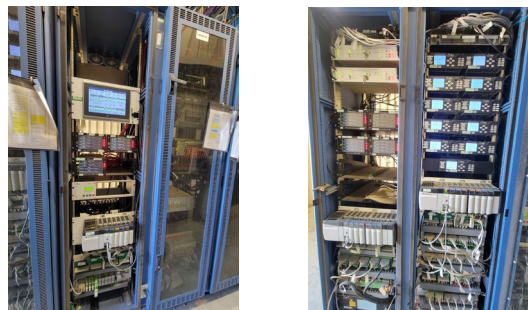
Figure 3: Typical LCLS-II Vacuum Controls Rack.
