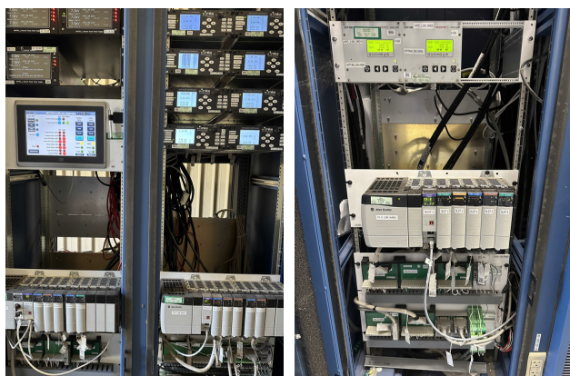
Figure 3: Example of sector controls rack installations.
