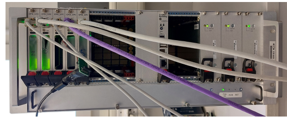
Figure 1: Picture of CPSI-S crate with 5 custom (UFC) cards inserted into the left most peripherally slots, a System Monitoring card just right of the middle and 3 redundant power supplies on the right.
