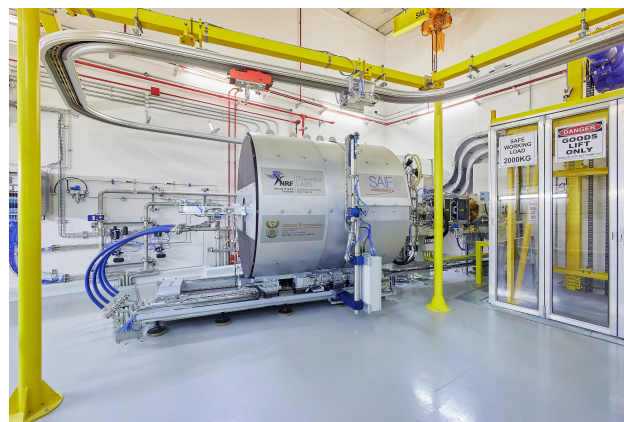
Figure 4: SAIF SR target station and transporter in vault.
