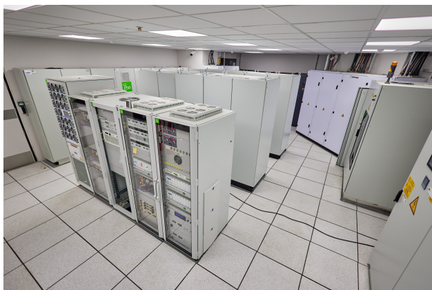
Figure 2: SAIF power supply and electronics room.
