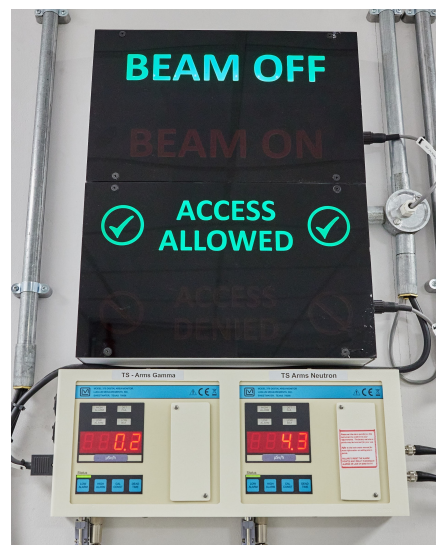
Figure 5: Electronic signage and radiation controllers as part of ARMS system.
