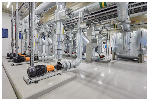
Figure 6: Chilled water plant.
