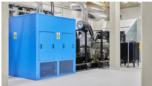
Figure 7: Diesel rotary uninterruptible power supply (DRUPS) installation.
