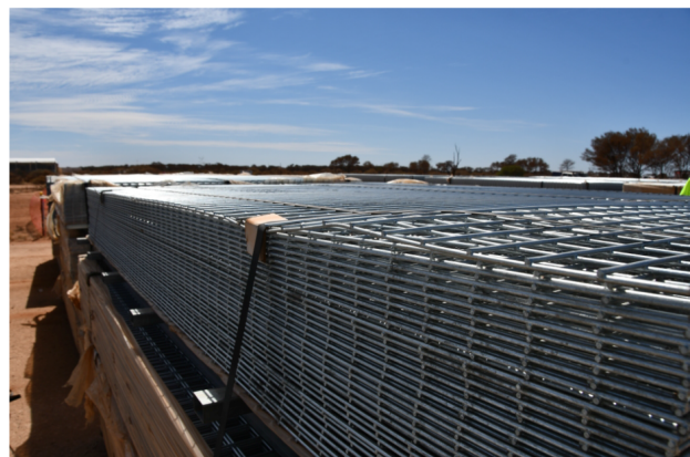
Figure 3: Recent construction pictures from the SKA-Low site. Left: A container of antennas; Right-top: Cable spools in the lay-down area; Right-middle: The partially completed AAVS3 station; Right-bottom: Wire mesh in the lay-down area.
